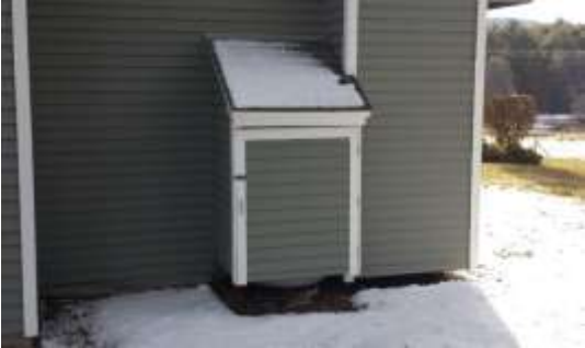
Unit 9 - Propane (Side)
