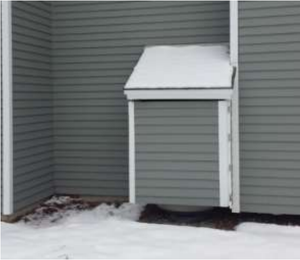
Unit 30 - Propane (Side)
