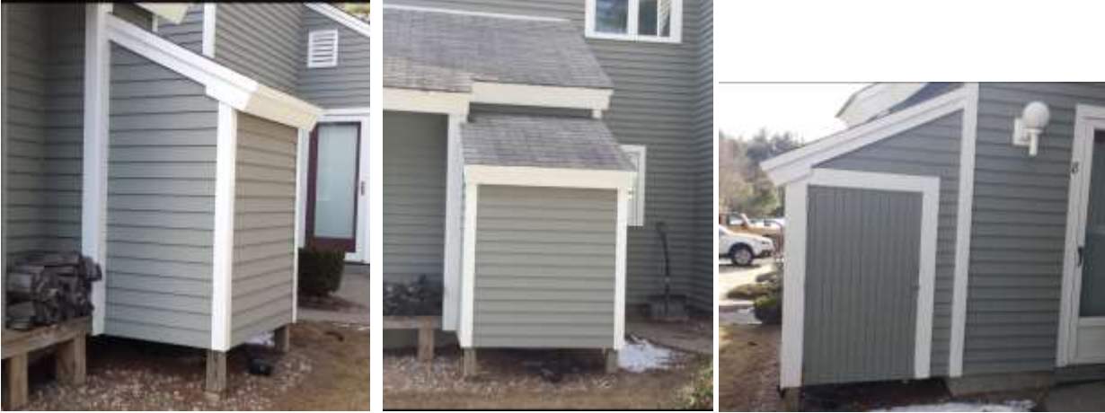
Unit 8 - Propane (Front)
